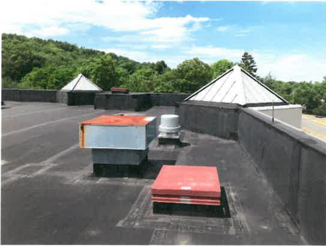
Photo 2 Oxidized roof top equipment
