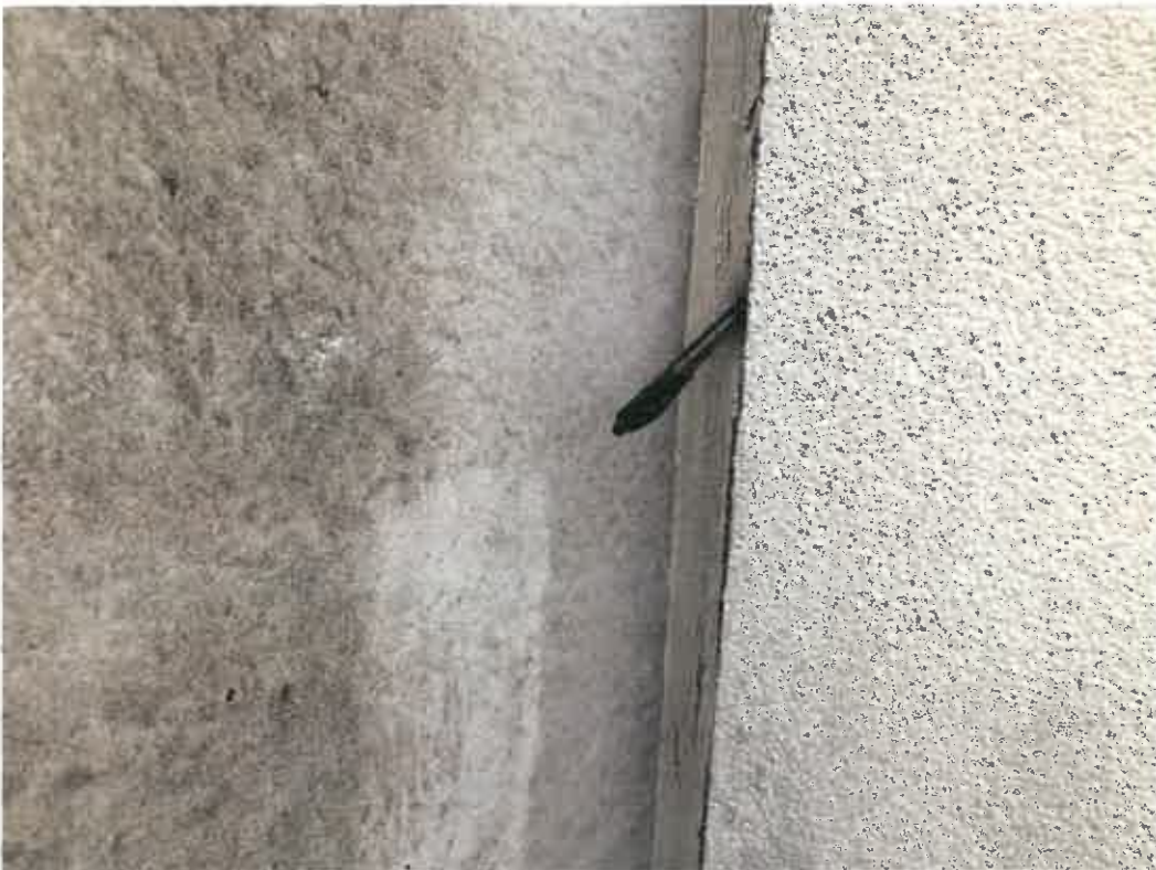
Photo 19 Deteriorated sealant at vertical joint
