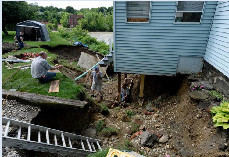
Photo 3a. 21 – Flood damaged home on North Street in Valley Falls, June 2014 (timesunion.com)
