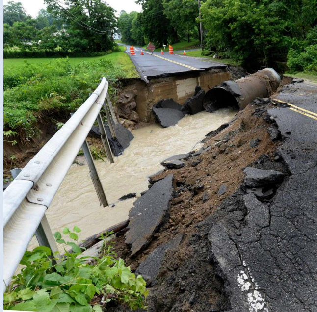
Photo 3a. 20 – Flood damage on River Road in Melrose, June 2014 (timesunion.com)
